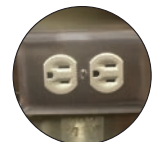
15A - 120V Duplex Receptacle Hidden Beneath Blender Shelf
